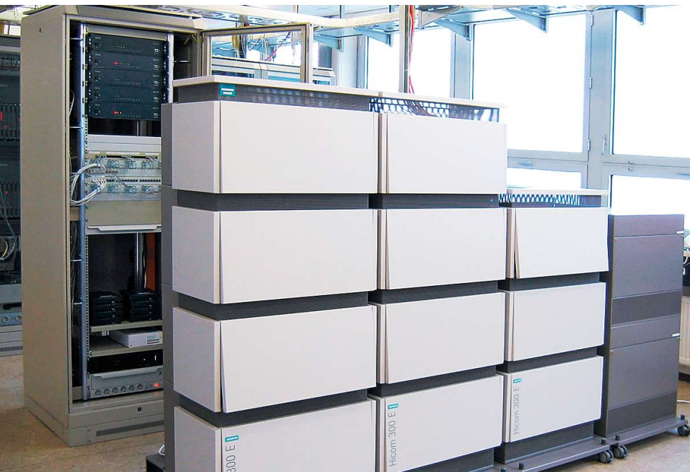
Secured communications at Rohde & Schwarz with a Siemens telephone system (front); behind it is the rack with the TopSec 730 encryption units.
